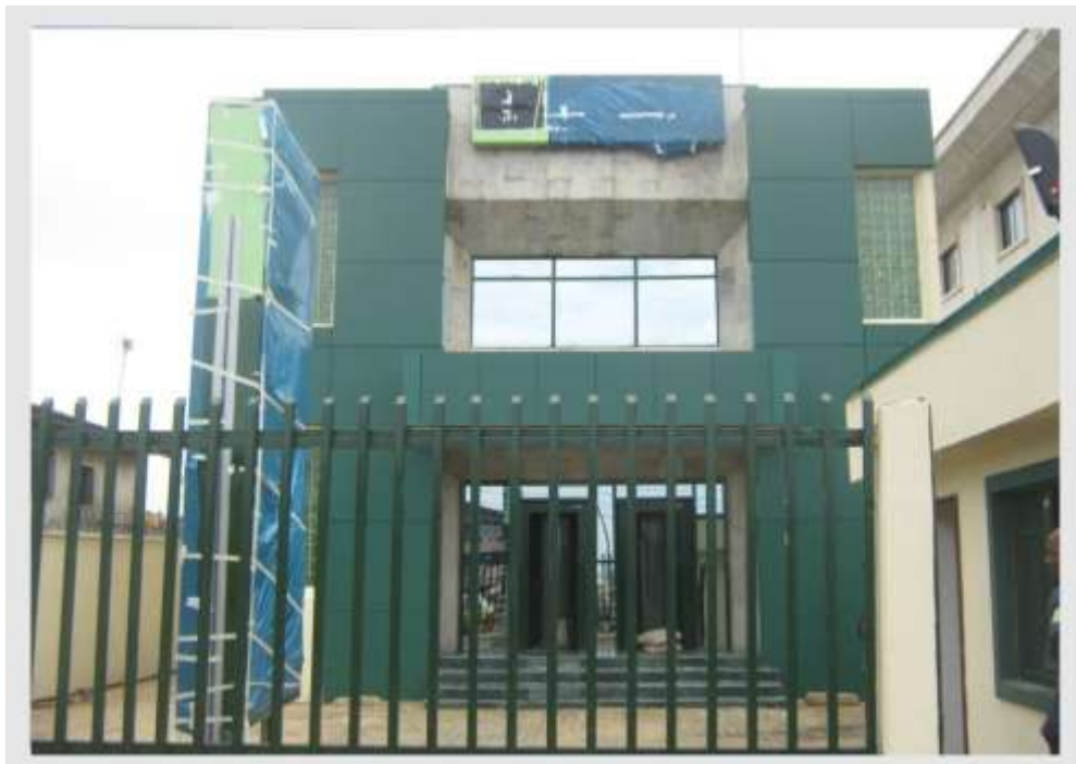
FIDELITY BANK PLC, IKORODU, LAGOS STATE
